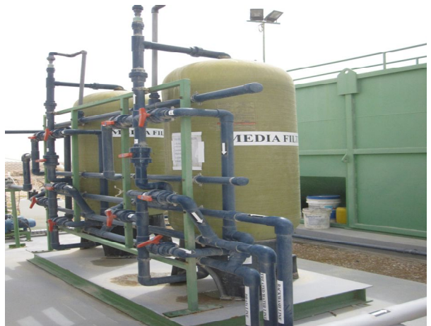
Filtration System of MBBR STP
