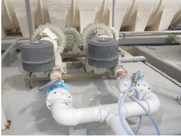
Aeration Side Channel Blower
