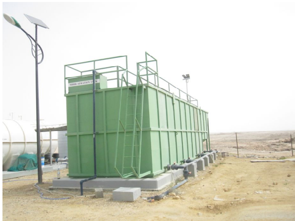
MBBR Aeration Tank
