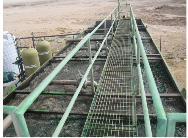
Aeration Tank with Bio Media
