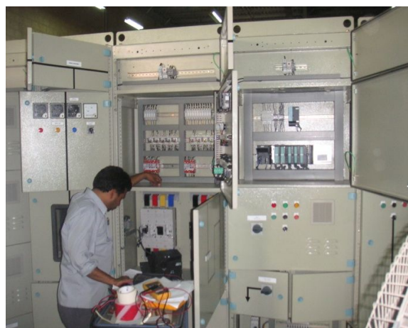
Fabrication and Testing of Automation Control Panel
