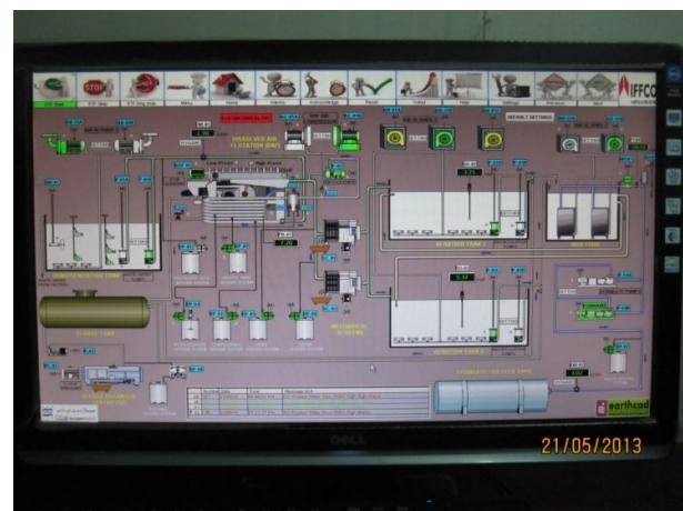
Desktop Based SCADA System at IWATER MBR STP
