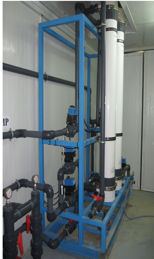
UF Module inside a 40 feet container in Duqm
