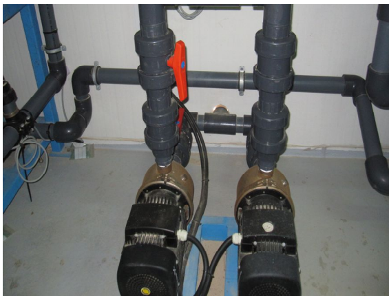
Feed Pumps to UF System
